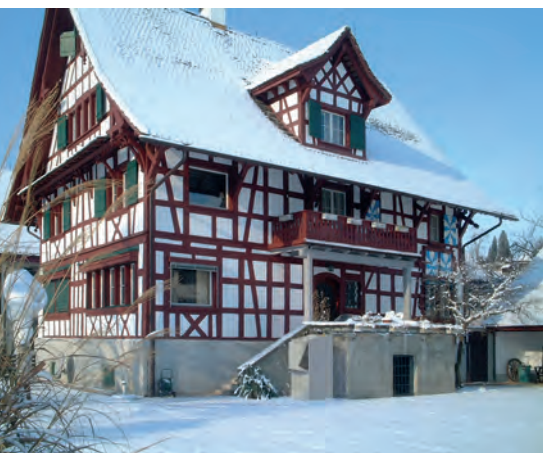
Historical single-family house with an outdoor air heat pump.
